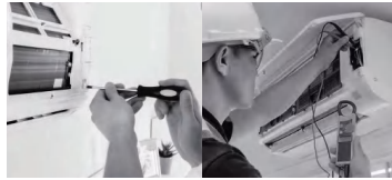
Complicated Wiring Steps Difficult Connecting
