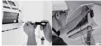
Complicated Wiring Steps Difficult Connecting
