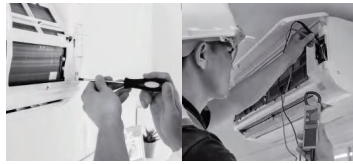
Complicated Wiring Steps Difficult Connecting
